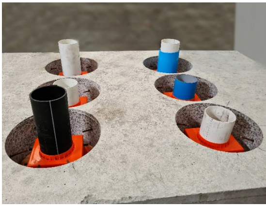
To ensure concrete does not fill into the collars, install a pipe former to the collar.
