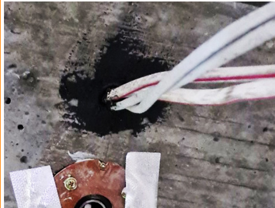
Once the slab has been poured and cured, simply backfill FyrePEX TM HP sealant into the service to a depth of 30mm.
