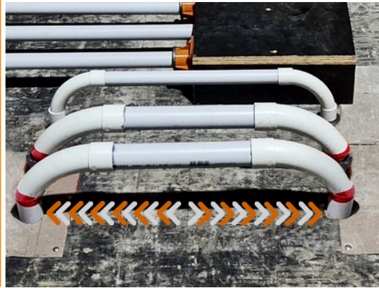
Depending on the required FRL the minimum distance the service must run through the slab changes to be compliant with the approvals.
