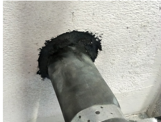
FyrePEX™ HP Sealant applied to a depth of at least 26mm from each side of the wall.
