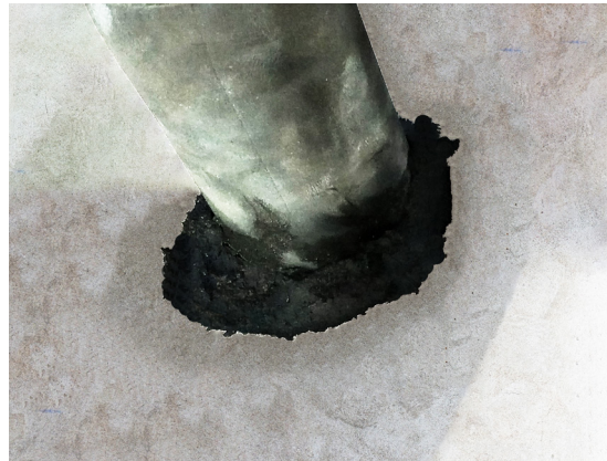
FyrePEX™ HP Sealant applied to depth of at least 60mm from top side of floor slab.
