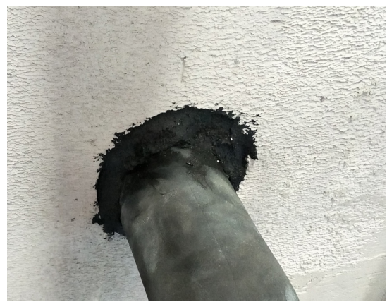
FyrePEX™ HP Sealant applied to a depth of at least 26mm from each side of the wall.
